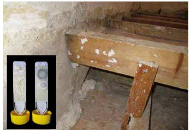
Microbial problems are often caused by moisture.
